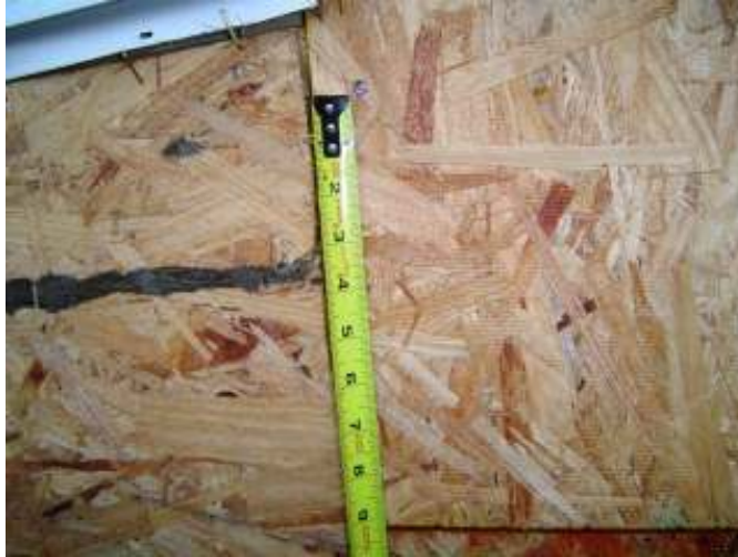
Example of incorrect nailing on OSB sheathing
