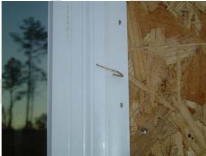
Window stapled through exposed finish
