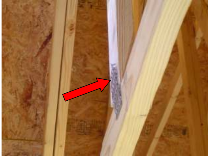
Damaged truss tie plate
