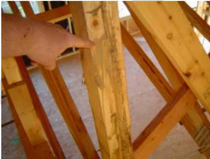
Improperly repaired cracked truss member
