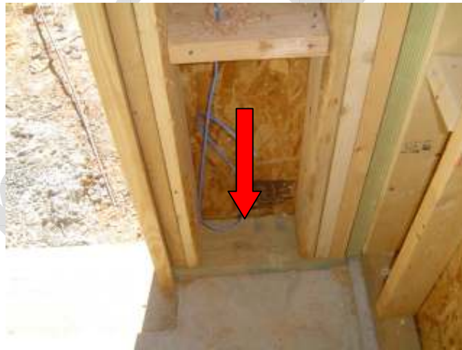
Anchor bolts missing at walls in garage example
