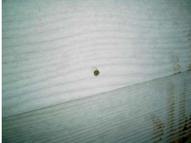
Overdriven nail in siding not properly repaired
