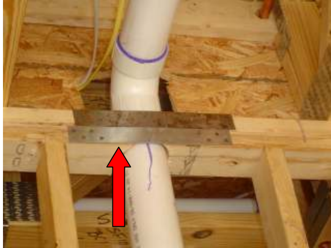
Shield plate does not extend two inches below top plate example
