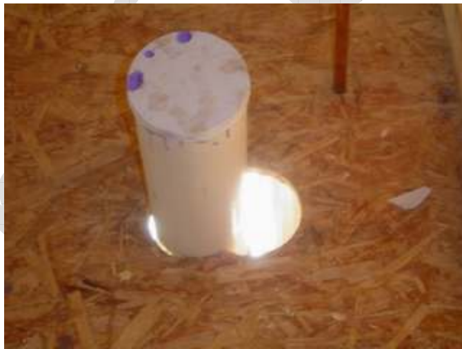
Fireblocking missing at plumbing penetration example
