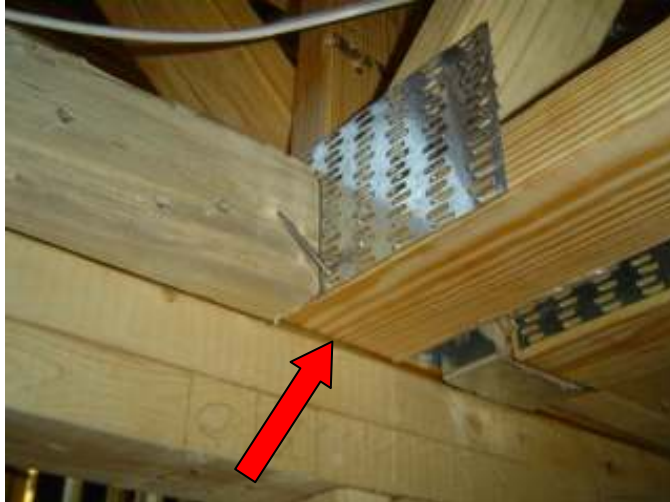
Floor truss no bearing on end
