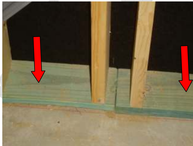
Foundation anchors not installed within 12 inches of ends of plate sections
