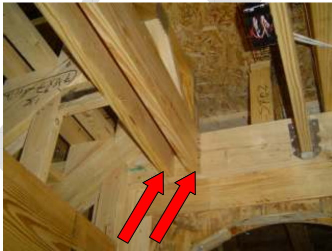
Examples of ceiling joists without proper bearing on ends
